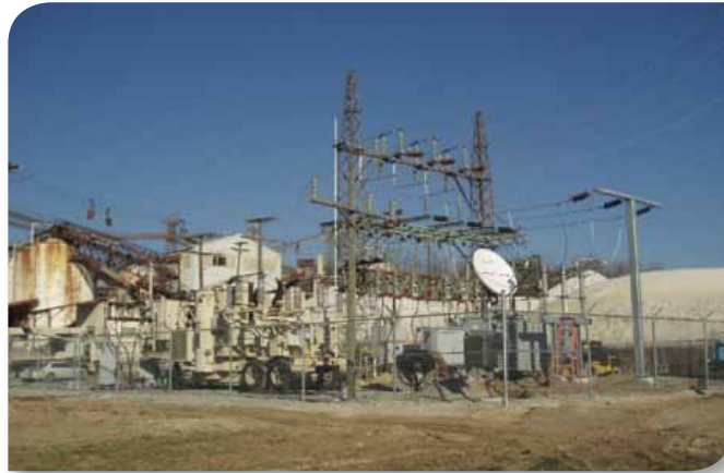
Example of satellite broadband at a power substation
